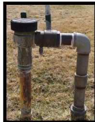
Pressure Vacuum Breaker (PVB)
